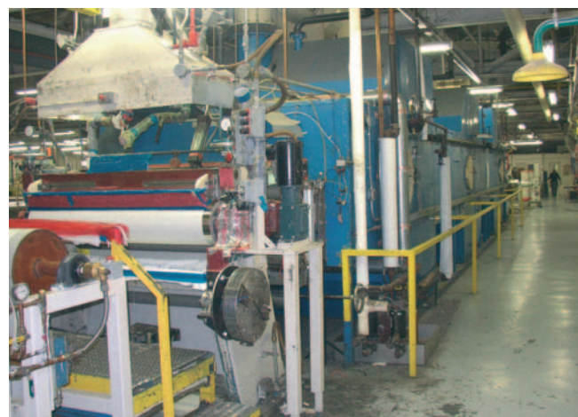
Adhesive coater at Ideal Tape Co (Lowell). 36m long, 3m wide, 5m high with 1.6m coat width.
