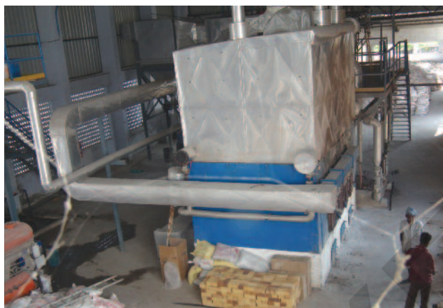
Wood and biomass steam generating plant.
