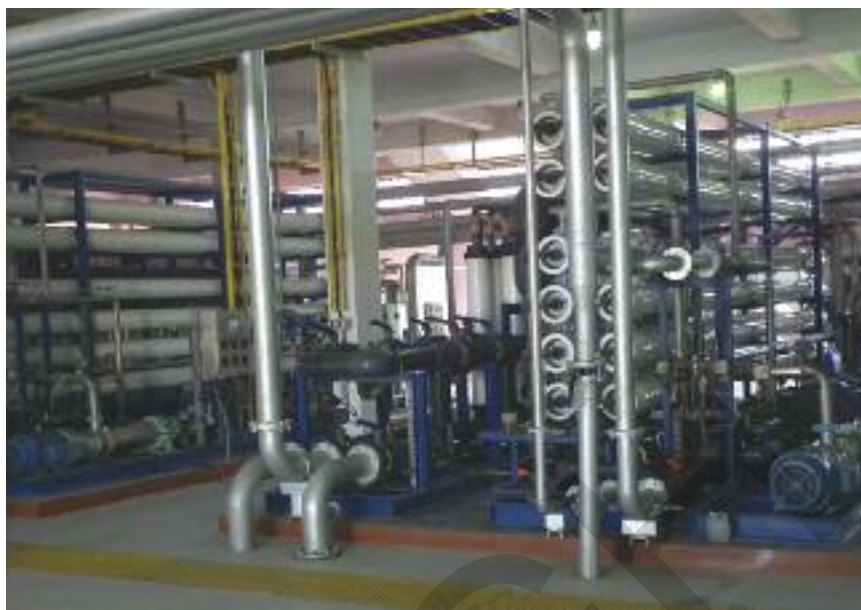
A process of reverse osmosis and evaporation/condensation enables 95% of tannery effluent entering the Ranipet CETP plant in India to be returned for reuse. CREDIT: WTP
